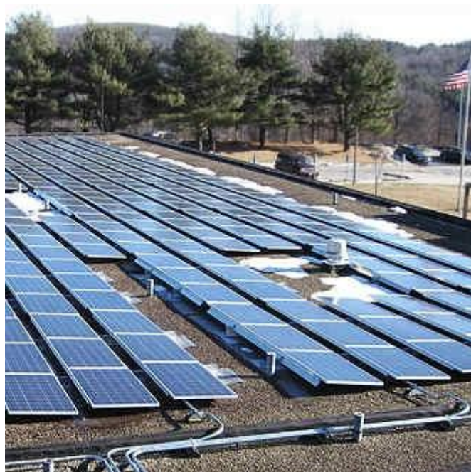
Fig. 10: Northwestern Regional No. 7 PV system
